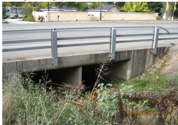
Photo 6. View of the culvert under Sunrise Blvd through which the unnamed drainage exits the Property.
